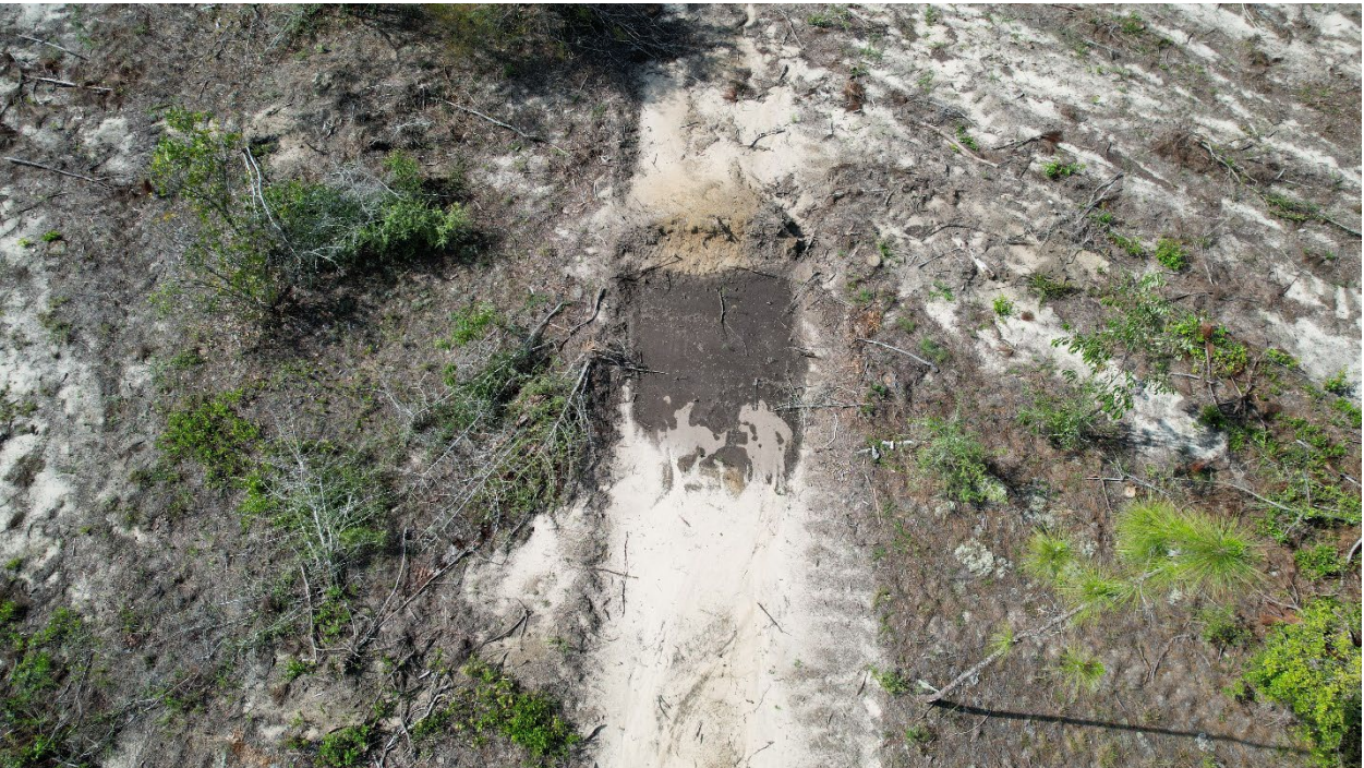
Image 9: Water bars on forest roads, a measure designed to channel runoff and minimize water accumulation.
